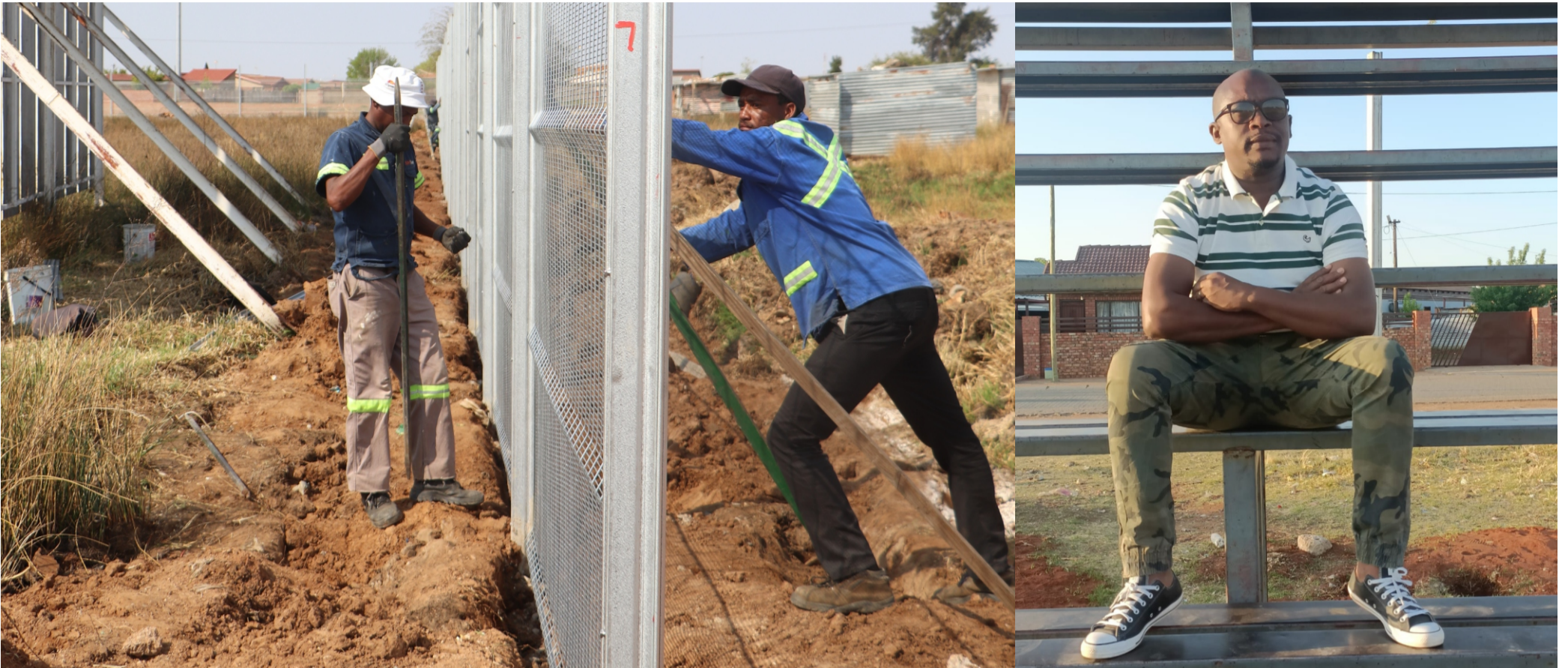
Building the foundation for future champions: Workers at Frank Foro Cricket Pitch
